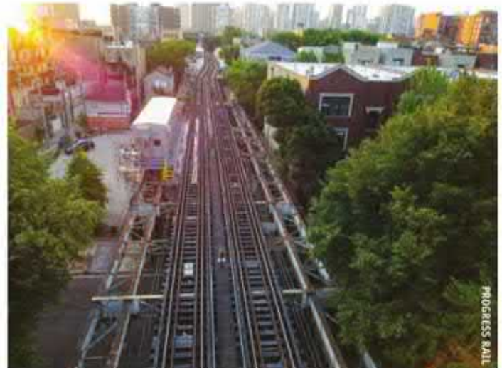
Progress Rail installed a signal bungalow as part of a larger project completed for a Chicago transit system.
