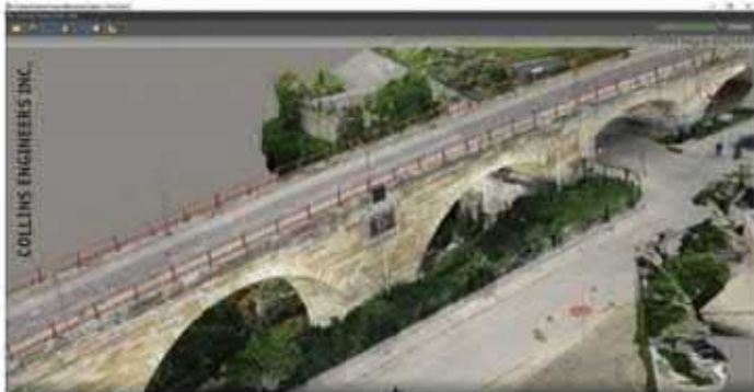
As part of the Stone Arch Bridge rehabilitation project in Minneapolis, Collins Engineers used Bentley's digital twin technology to transform bridge inspection.
