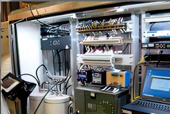
PTC Communications Lab
